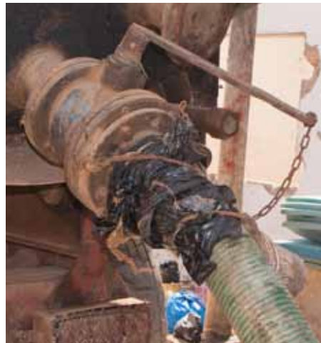
Figure 4.13 Example of an improperly maintained hose held together with plastic bags and twine (photo: David M. Robbins).
