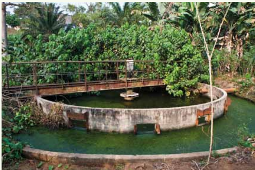
Figure 17.3 A non-functioning treatment plant in Yaoundé, Cameroon (photo: Linda Strande).
